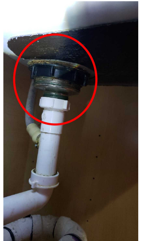
Corrosion and deteriorated drain fitting
