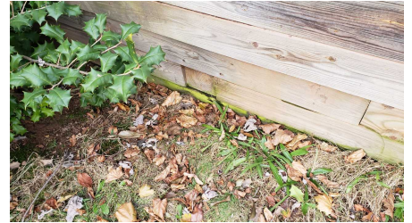
Direct wood to soil contact will eventually rot away wall
