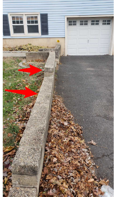
Wall is bowing outward
