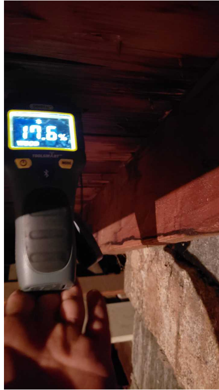
High moisture reading
