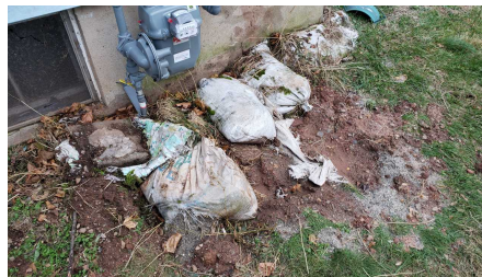
Proper compaction is suspect, observed leak in basement
