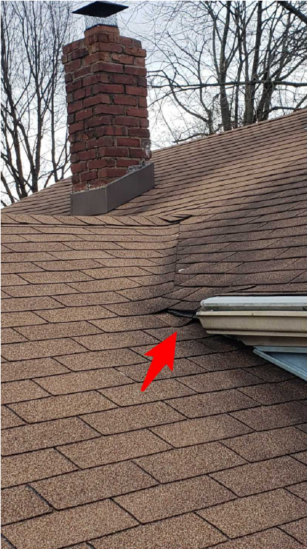
Pitched onto roof. In need of repair. Leak observed below this area
