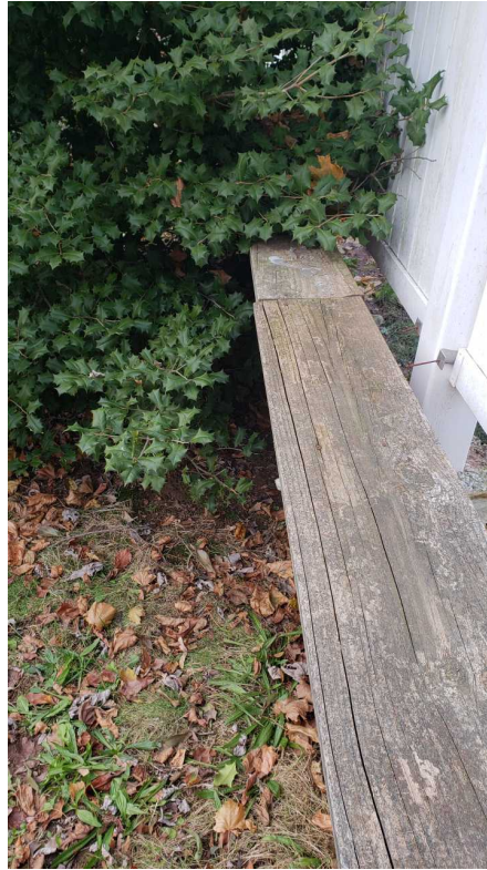
Wall is bowing
