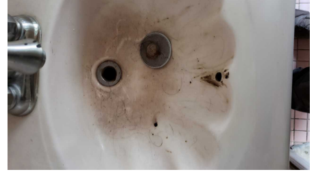
Clogged and stained
