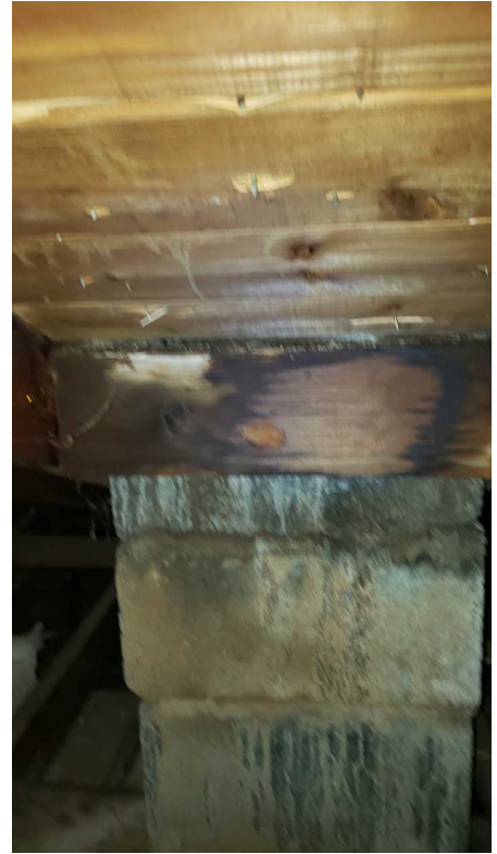
Evidence of previous leak around chimney
