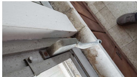
Windows in the rear sunroom are difficult to open
