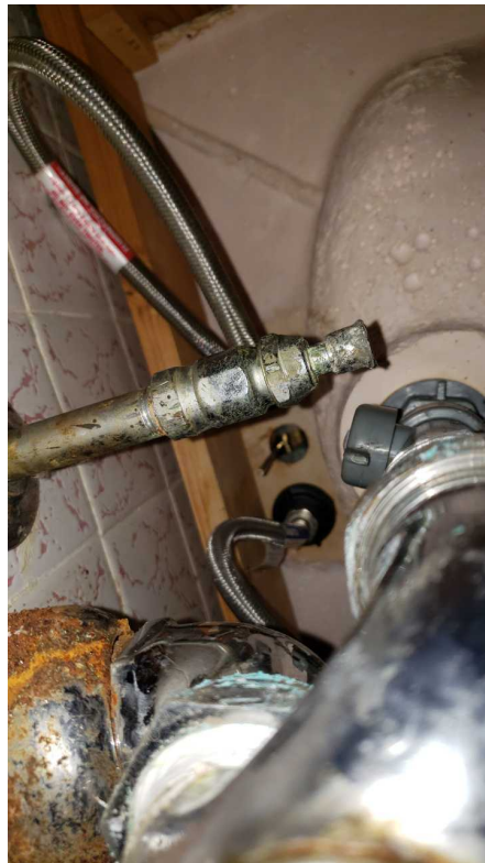
Corrosion on drain
