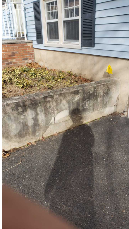
No weep holes and spalling
